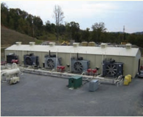
The Clarksburg Compressor Station was completed in November 2010.
