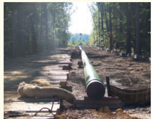
The Monroe Gas Storage Facility was completed in November 2009.
