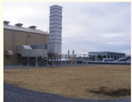
The Bald Knob Station Expansion was completed in 2009.
