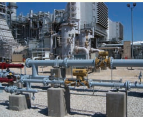
The Brazos Compressor Station was completed in June 2010.
