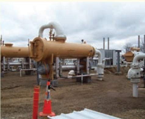
The REX Measurement Facilities were completed in 2009.
